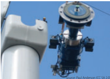
This huge 12 ton gearbox and disk brake assembly is lifted with a crane to a height of 60 meters to be mounted in this wind turbine nacelle.
