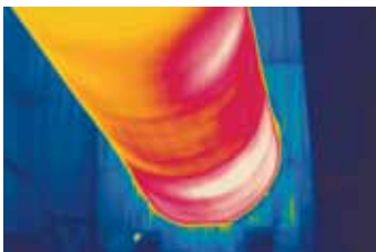
Breakdown of refractory on a rotary cement kiln
