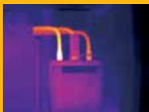
Poor connection and internal damage
