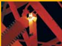
Incorrectly secured connection
