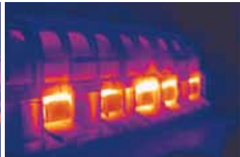
Refractory insulation defect
