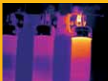
Internal fuse damage
